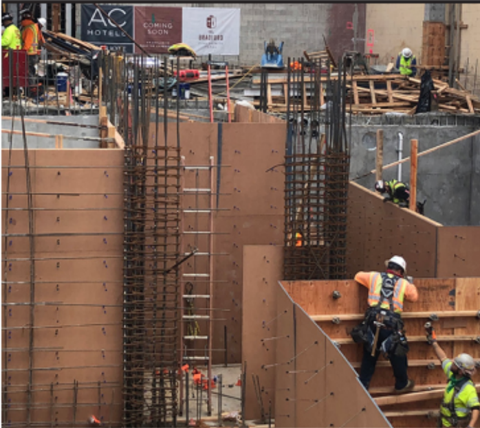
THE $65 MILLION AC BY MARRIOTT SAN DIEGO PROJECT IS LOCATED IN THE HEART OF THE CITY'S GAS LAMP DISTRICT. THE BRIAD GROUP IS AIMING FOR COMPLETION IN MARCH 2021.
